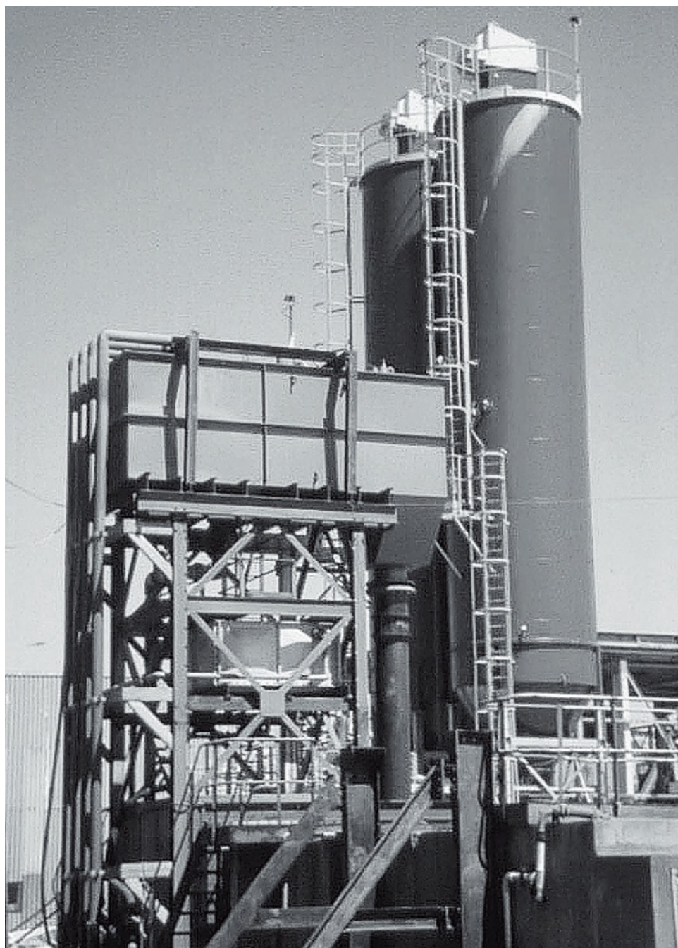
Figure 4.4: Lime silos at a high flow-capacity (8–15 MI d -1 ) conventional ODAS mine water treatment plant (former ‘temporary plant’ at Wheal Jane, Cornwall, UK). For a discussion of the evolution of treatment technology at this site, see Lamb et al. (1998) and Worked Example 4.3. (Photo: P. Younger).
