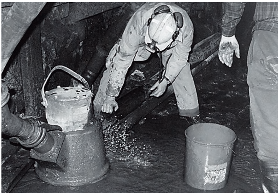
Figure 3.28: A small underground dewatering sump: the main pumping lodge on the 295 Level, Frazer's Grove Fluorspar Mine, Weardale (UK). John Evans checks the end of a rising main feeding into the sump, whence the large Flygt™ pump lifts the water to the next sump in the system. For details of the overall dewatering system in this mine see Younger (2000b). (Photo: A. Doyle).
