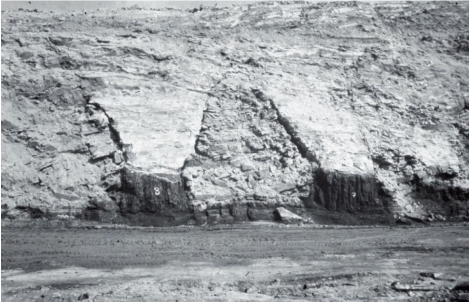
Figure 1.12: Two old mine roadways dating to the late 19th Century, which have subsequently closed entirely by plug failure of the overlying sandstone. (High Main Seam, Morrison North Pit, Co Durham (UK)). These were exposed during working of the Chapman's Well Opencast Mine in the early 1990s. (Photo: A. Witcomb).
