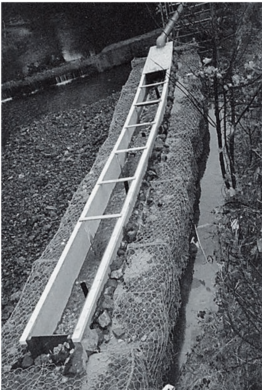
Figure 5.6: ( See opposite for 5.6B ) A – Pilot-scale saturated-flow SCOOFI reactor at Skinnigrove, Cleveland (UK), as described by Younger (2000d). The mine water moves through the blast-furnace slag held in the gabions, and iron is removed by surface-catalyzed oxidation of \text{Fe}^{2+} . B – The prototype unsaturated flow SCOOFI reactors at Kimblesworth, County Durham (UK), as described by Jarvis and Younger (2001). The reactor comprises two towers filled with lumps of plastic and/or blast furnace slag (both of which have high specific surface areas).
