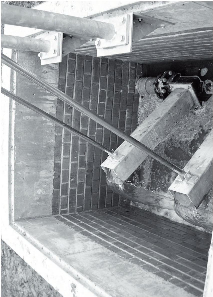
Figure 5.15: Adjustable-angle elbow joints forming a simple but effective means of controlling water levels in a constructed wetland. If the angle of the decanting pipe is changed, the water level in the wetland upstream must also change to maintain the same flow rate. (Photo: P.L. Younger, with the permission of the site owners, Northumbrian Water Ltd).
